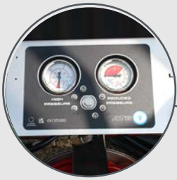
Control Panel Gauges & Whistle
